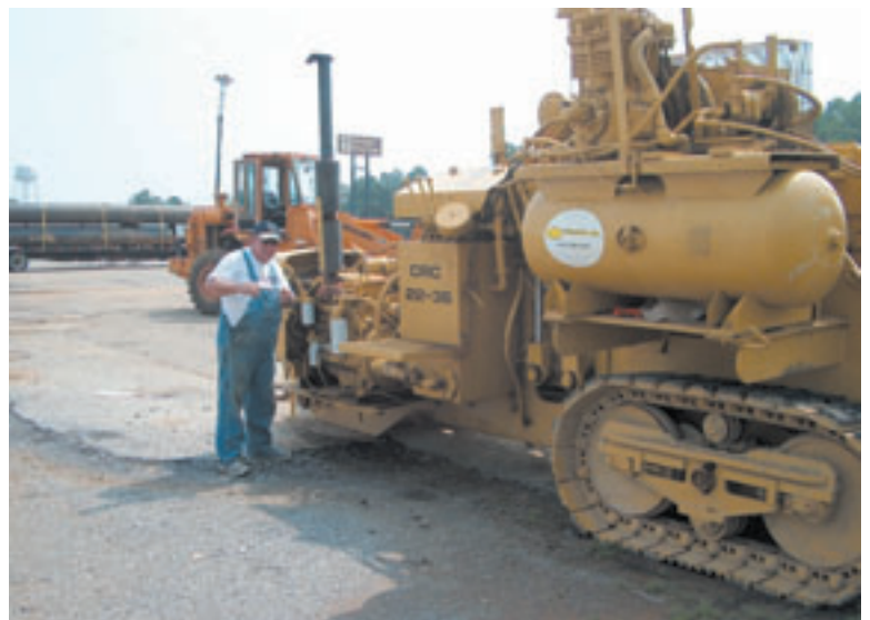
Carl Hylton -- co-owner of Alpha Pipe Company, Inc. -- oversees pipe straightening at a temporary job site.
